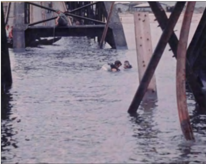
SOUTH VIETNAM--SEABEE DIVERS INVESTIGATE THE EXTENT OF DAMAGE DONE TO A BRIDGE BY RECENT VIET CONG SABOTAGE.
